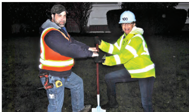
From left, Project Superintendent Tim Jacobs and Oregon Alpha Chapter House Corporation President JANET UHLENHAKE CLAY, Oregon Alpha, break ground on the chapter's building addition.
