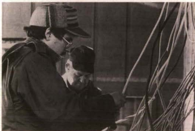
Maintenance men Jeff Monhollen and Zanley Watson install electrical wiring in the wood studio addition.
