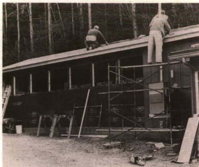
The new woodworking studio as it was in progress during the winter.
