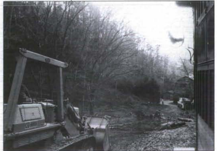
Preparation for construction of the new dorm began in November. This view shows the construction site above the Red Barn.
